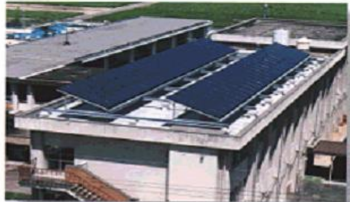
Solar cell capacity: 20 kW
